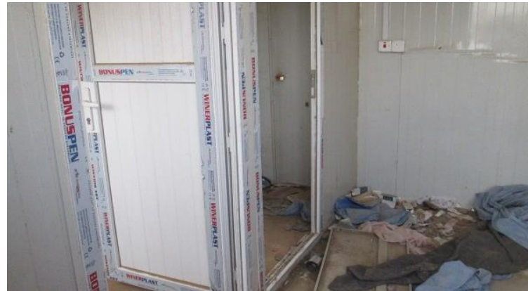
An example of WASH infrastructure in Primary Health Care Centre damaged during the liberation operations of Wanna Sub - District, in Northern Ninewa, Iraq
