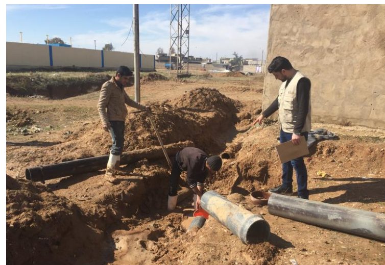
Step by step the water supply network in Tal Afar is repaired (September 2018)
